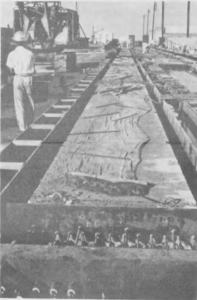
EIGHT SLABS are fabricated at a time in each of the stress beds. They are kept covered and damp during the three-day curing period.
